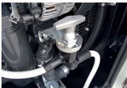
Batterieschalter Battery isolator switch
