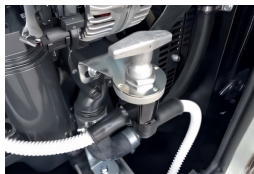
Batterieschalter Battery isolator switch
