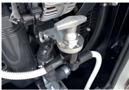
Batterieschalter Battery isolator switch
